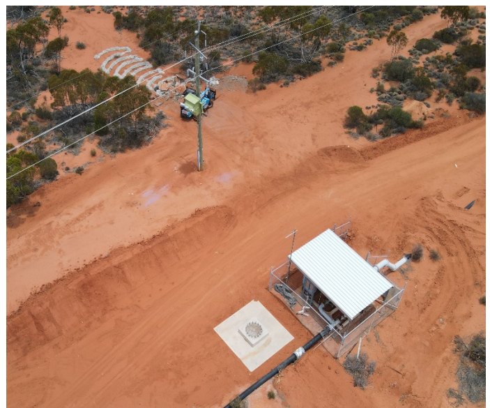
Battery bore field process water transfer station
