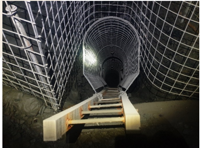
Emergency escape ways reinstated
