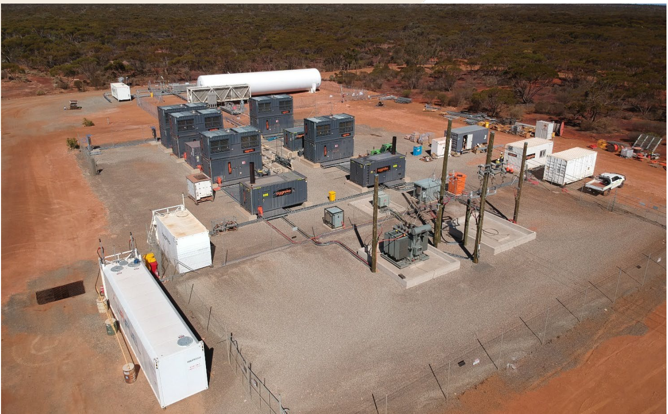
New Power Station with LNG facility in background pre-commissioned
