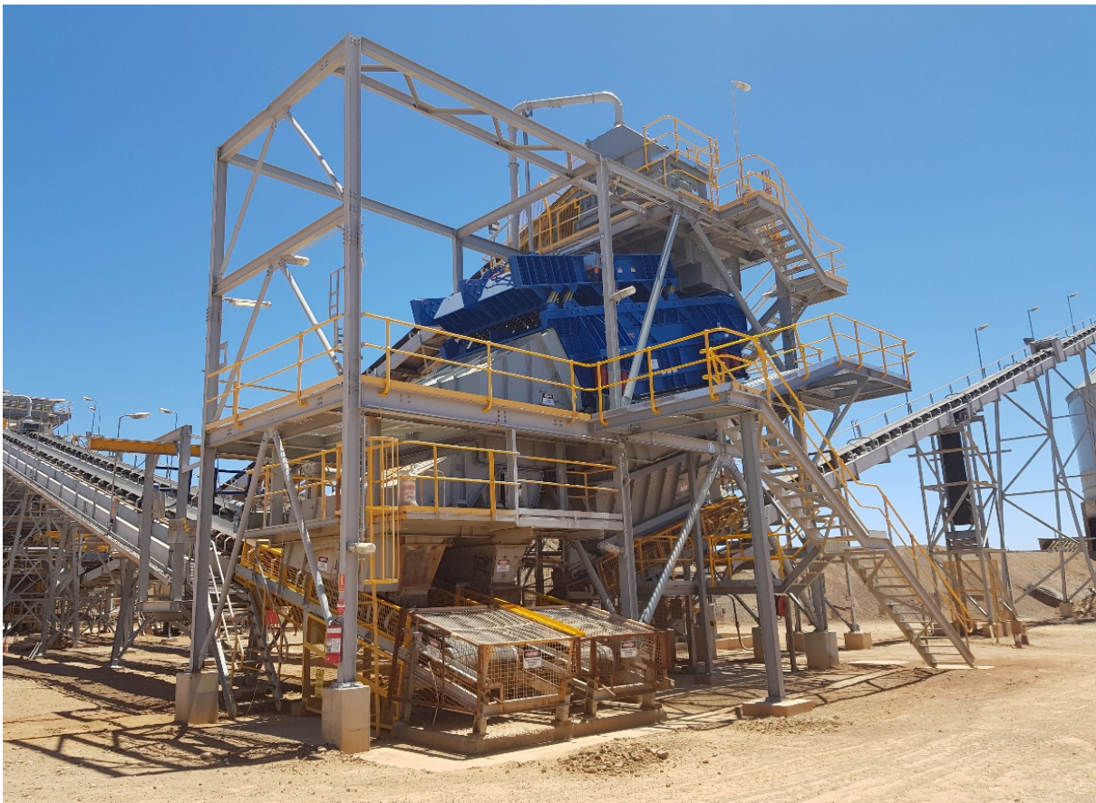
New product screen installed in December and dry commissioned
